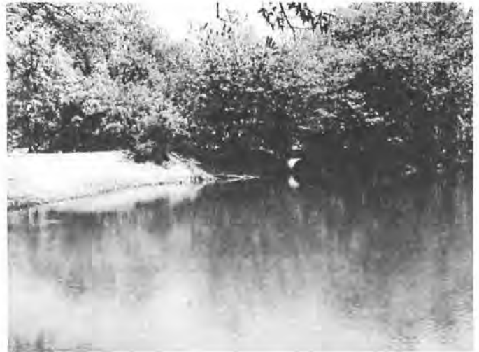
The new culvert between the cement plant pond and Juno Pond. (photo by Jon Seymour)
