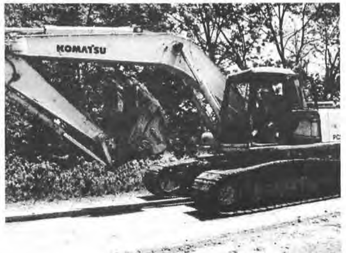
It takes some large equipment to install culverts (photo by Jon Seymour)
