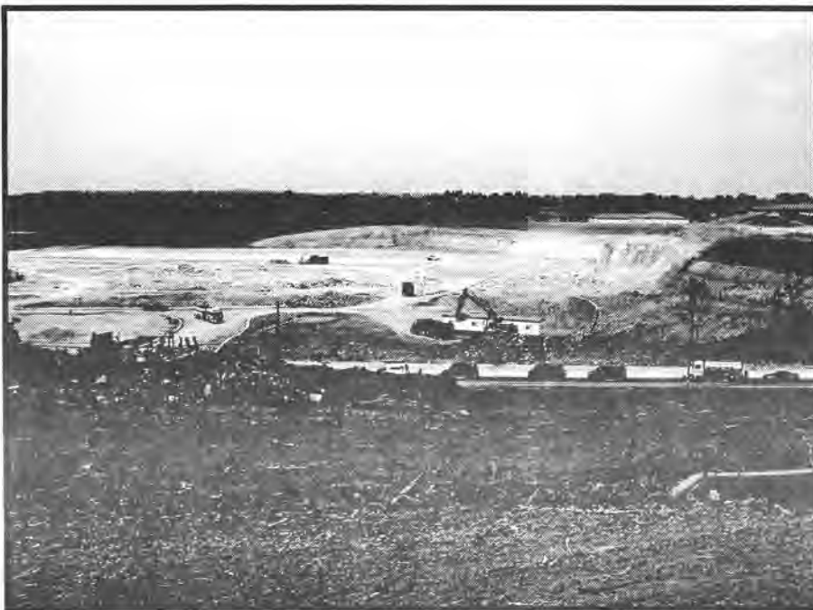
Figure 3 - the developer removed all trees as well as the steep hillside and streams to create a flat 37 acre site for the Kohl/Meijer's retail complex at the I-74 Harrison/Rybolt interchange. In the foreground, a 10 acre hillside was leveled for three fast food restaurants. These sites drain into Taylor Creek which in turn flows into the Great Miami (Photo by Roland Johnson)
