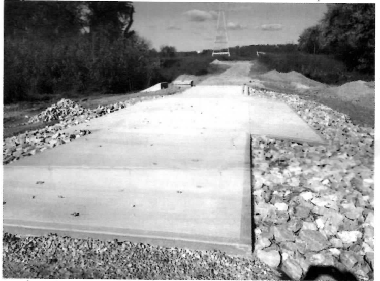
Concrete spillway with rip-rap cover on the sides for erosion protection. (photo by Jon Seymour)
