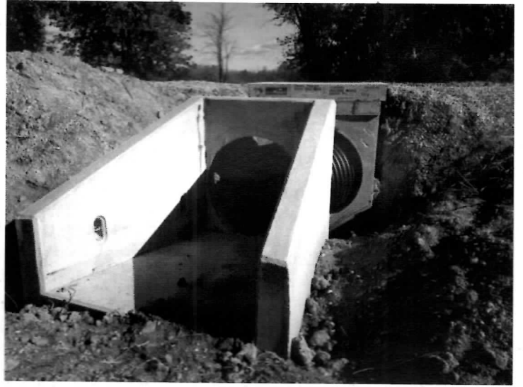
The large culvert box under the new raised road/dam. The square box behind the outlet contains the water control structure.
